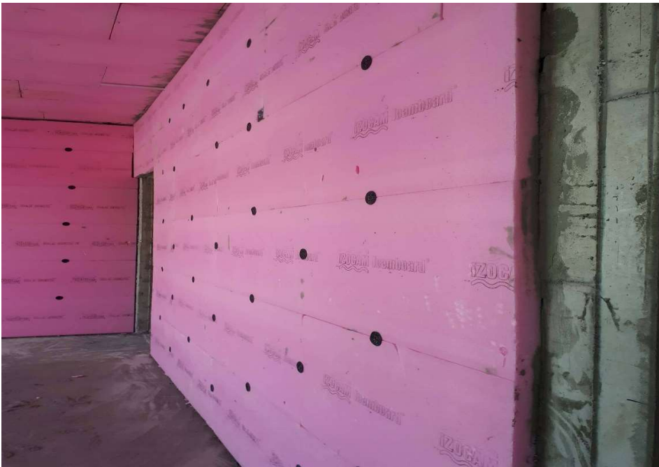
Using Extruded Polystyrene ( XPS ) foam for insulation from outside of the building
